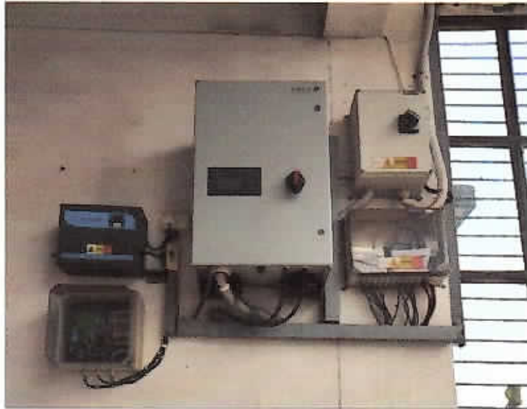
Solar Inverter and Metering
