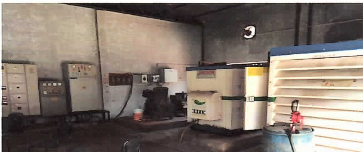
Electricity Generator Room
